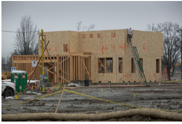
Businesses and residential homes in the Coffey Park neighborhood slowly move through the rebuilding process after a wildfire swept through Santa Rosa, California. Construction costs reportedly doubled after the fire. Photo by George Rose/Getty Images
